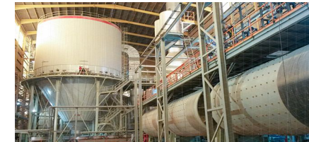
Work process: «Work involving exposure to respirable crystalline silica dust generated by a work process»
